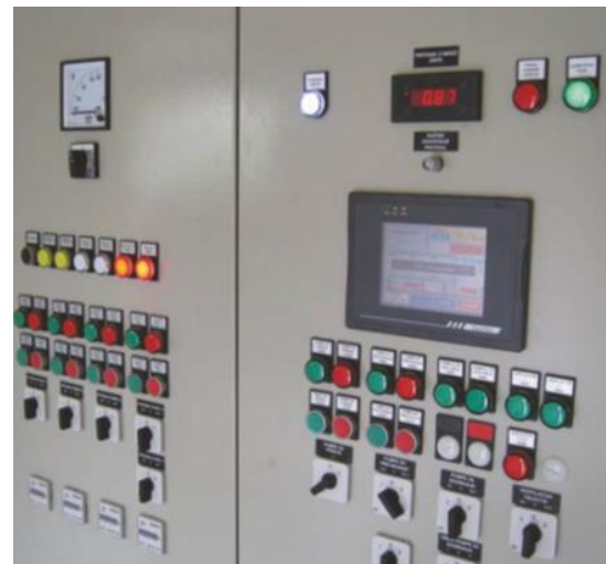
Figure 3. Electrical cabinet with touch screen panels
