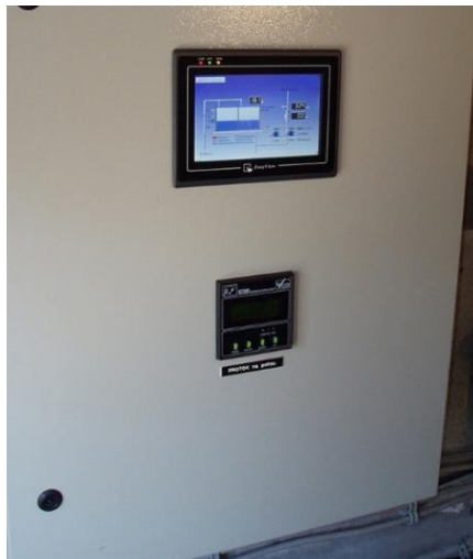
Figure 2. PLC with electrical cabinet
