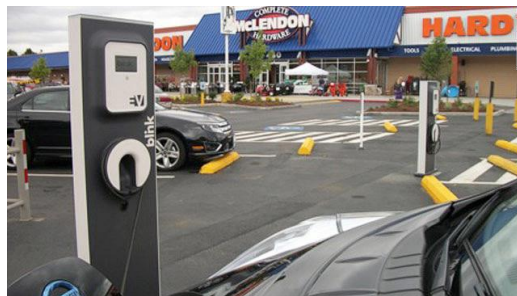
Figure 2. Example of a charger in front of a shopping center [4]
